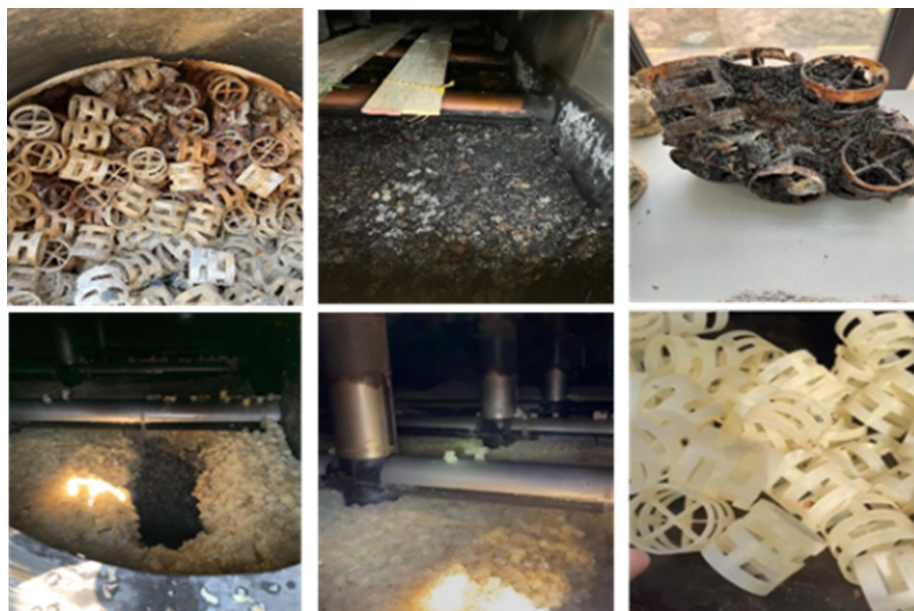
Figure 44 Ball Ring Before and After Cleaning
