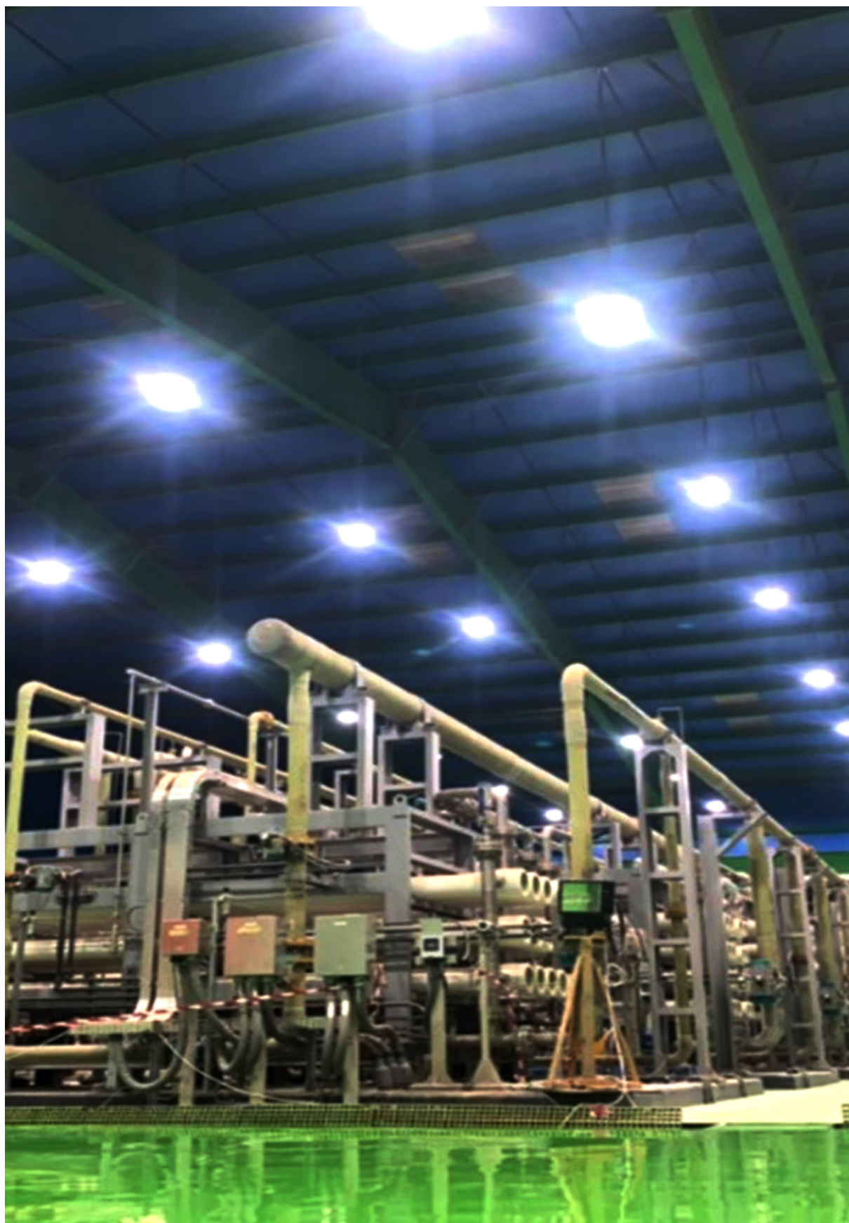
Figure 57 Shoaiba NF-Mg plant
